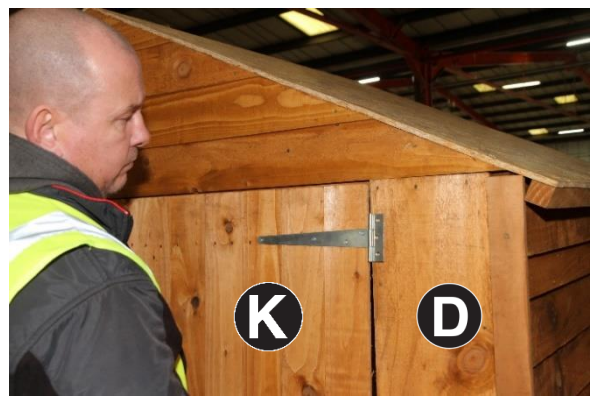
25. Attach Part K to Part D using 25mm screws leaving a 3mm gap from top to bottom along the side and a 6mm gap at top of door.
