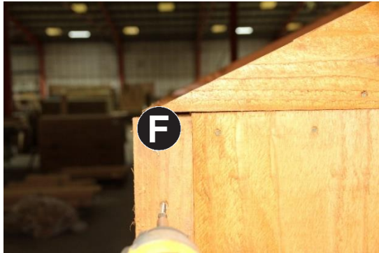
19. Fix Part F to all four corners of the shed leaving 10mm space from the top using 3no 40mm per corner top, bottom and centre.
