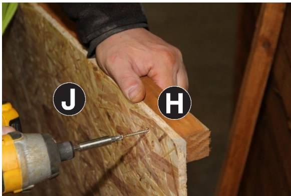
27. Attach Part H to Part J to the longest length flush with edge leaving an evenly spaced gap either end. Fix together using 4no 40mm screws. Repeat on all four panels.
