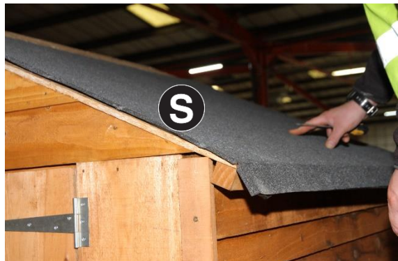
42. Cut Part S to three equal lengths and place on roof as per image with overlap.
